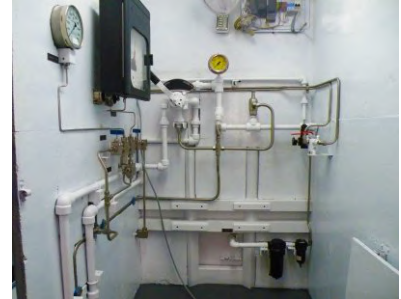
Workshop with test unit, Baker vice and chain hoist
